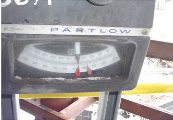
Steam Supply Pressure (600 PSI)
